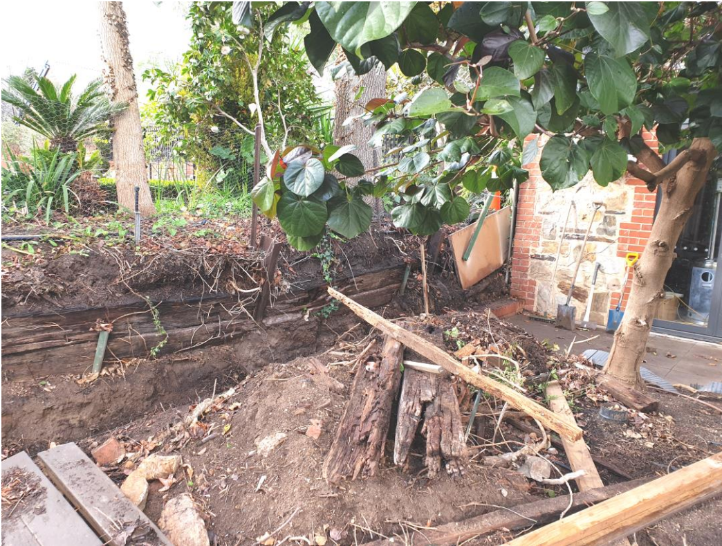
Photo 3 – Southern portion of area where retaining wall and fence proposed, taken from 36 Mills Terrace
